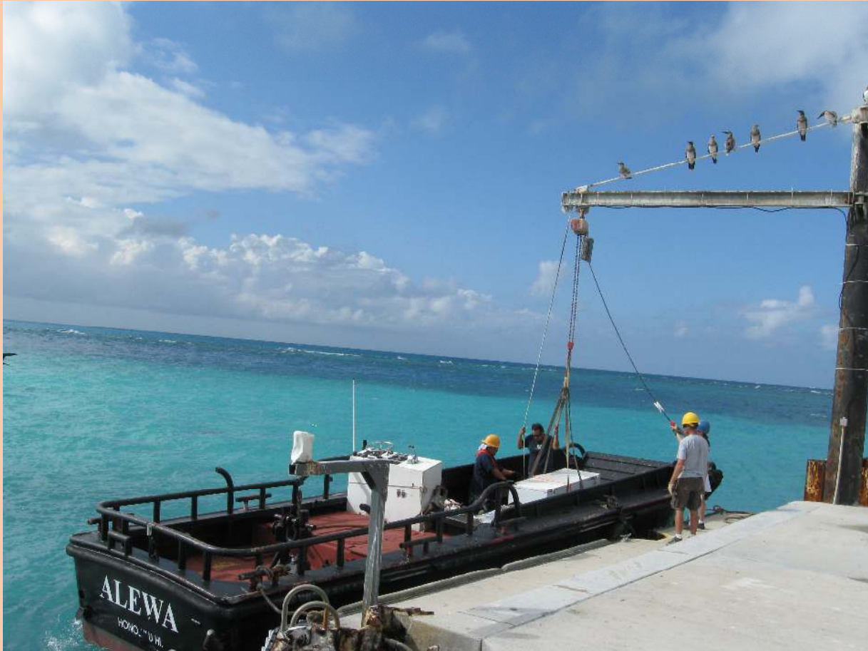
Equipment being off loaded on a Nexgen Energy Systems, Inc., photovoltaic project for the USF& Wildlife Service on a Pacific island 500 miles west of Honolulu, HI
